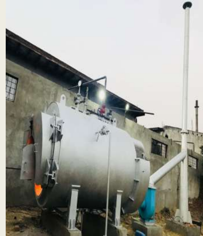
Two ton Thermax Multipack steam boiler.
